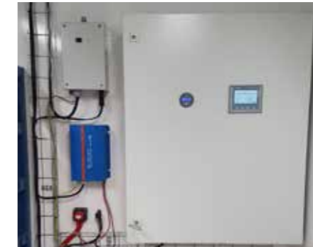
Energy Management System
