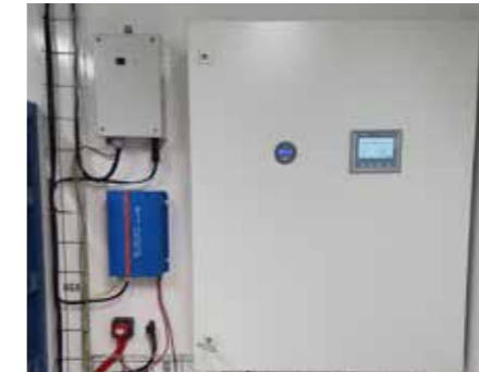
Energy Management System
